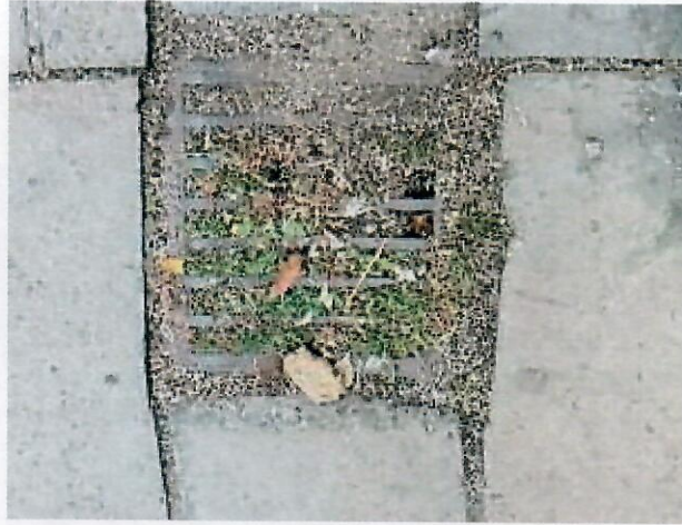
Blocked drain High Street
